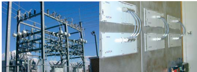
CTO 69 kV installed at Kunitz substations for LCRA, USA
