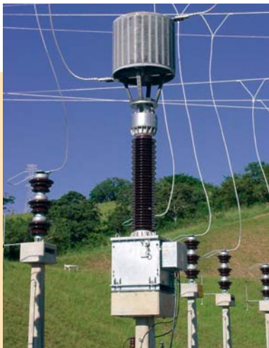
Vertical pedestal A line trap mounted on CCVT
