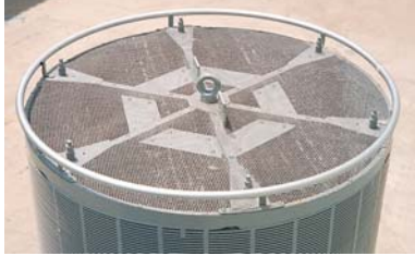
Details of line trap showing bird barrier, crossarms and corona ring
